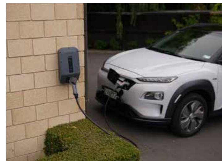
Modern home electric vehicle charging infrastructure (Image credit: Ed Harvey)
